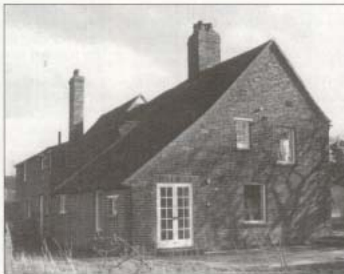
Rewindowing of the west gable - only the small window is original; the lower picture window replaces a 19th century sash, and the doors and upper picture window are new
